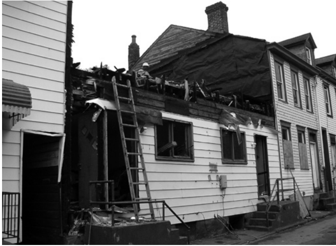
Lawrenceville United and its partners make a critical investment in the community by demolishing and converting crime-ridden, vacant and abandoned properties into new affordable housing.
